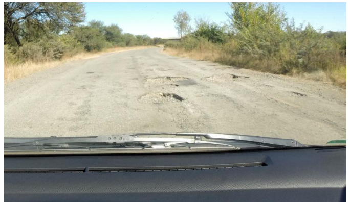
Fig. 1. Example of potholes in a road
